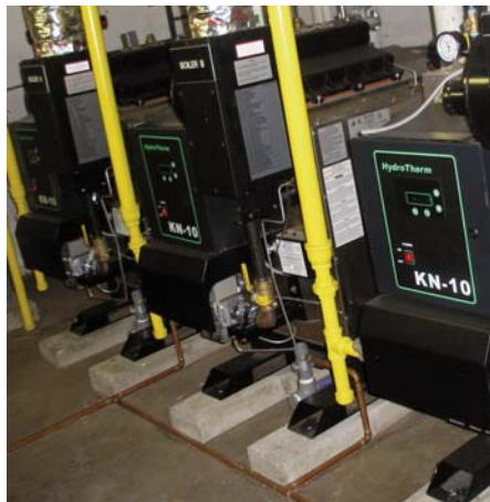
KN-10 boiler installation at The James (Major) Adams Community Center in Chicago.
