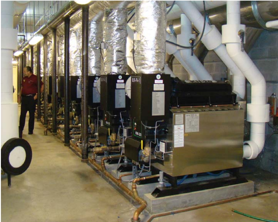
The KN-20 boilers are tasked with providing domestic hot water, kitchen and laundry hot water, hydronic heating, pool heating and re-heat/humidity control for the entire hotel.
