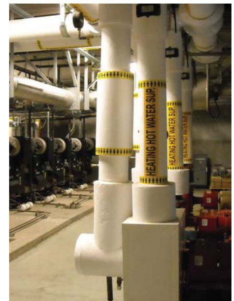
The KN-20 boilers are tasked with providing all of the hot water necessary to heat the physical space and aquatic exhibits in the Academy.
